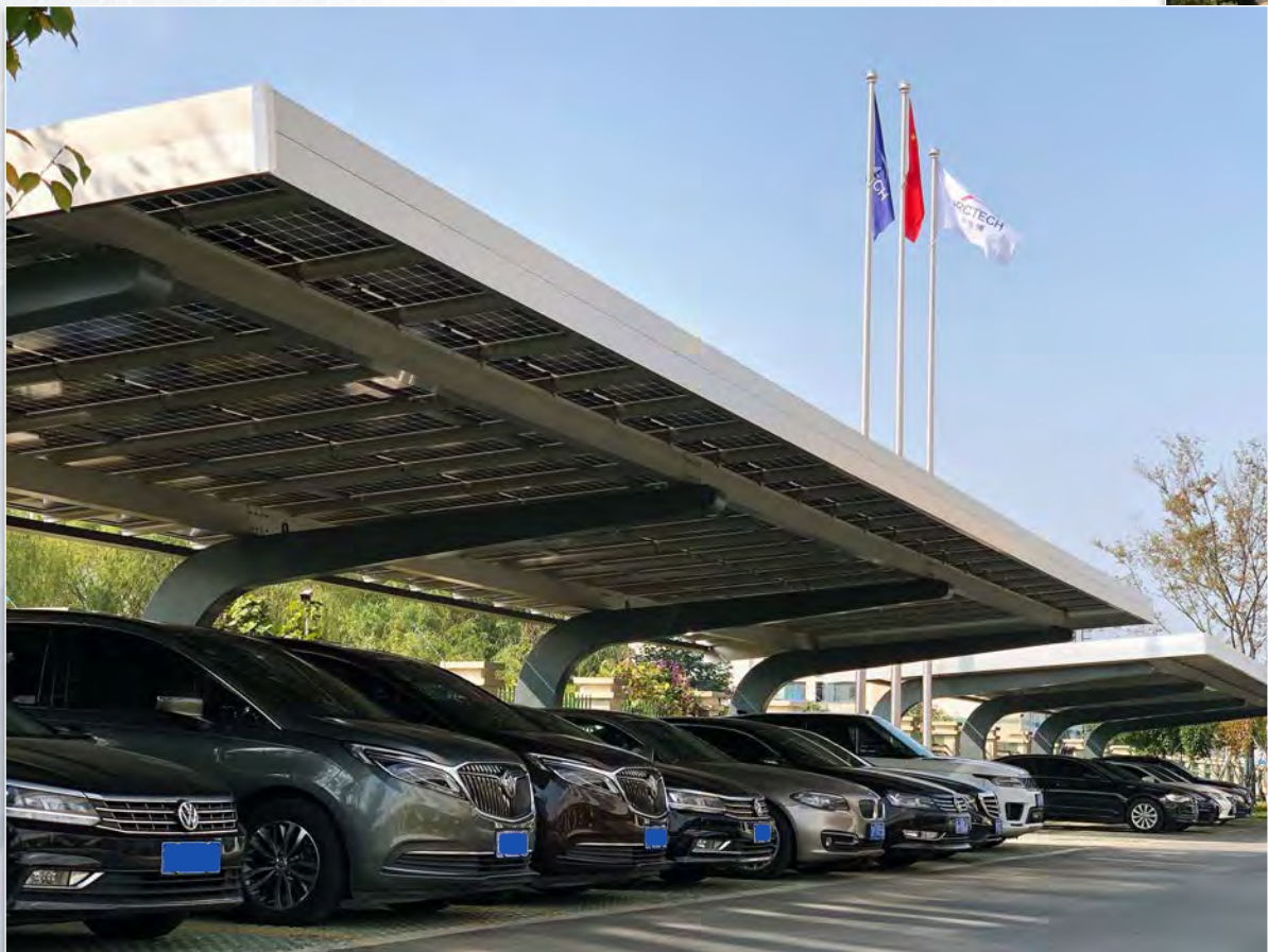
Solar carport with EV charger
